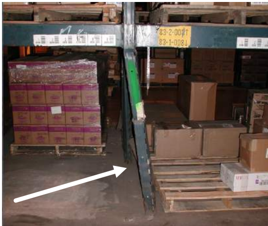
Damaged upright column
