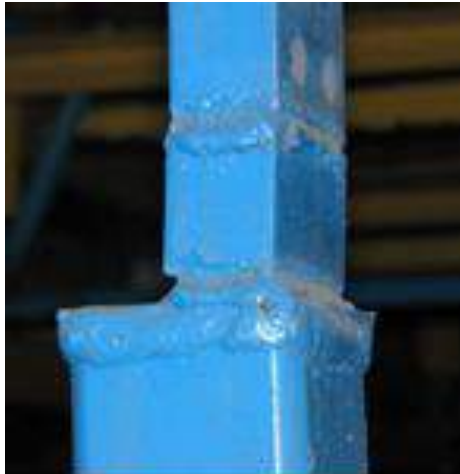
Unsafe field welding repair
