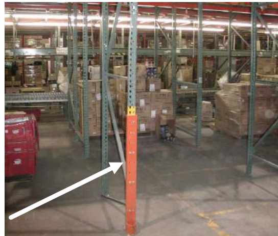
Damaged column with home-grown repair
