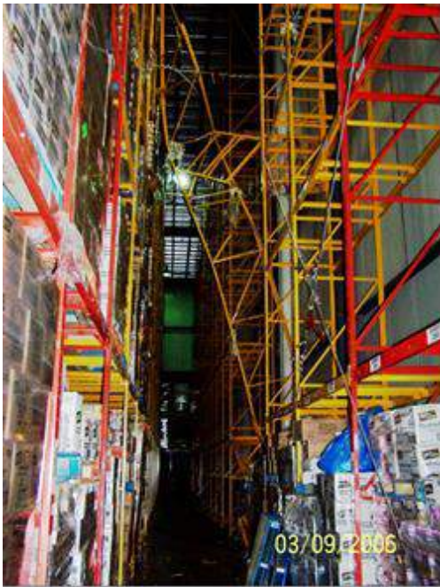
Rack damage was ignored
