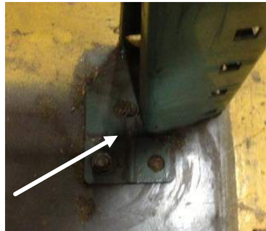
Sheared anchor; footplate separated from column
