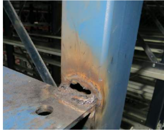
Defective field welding
